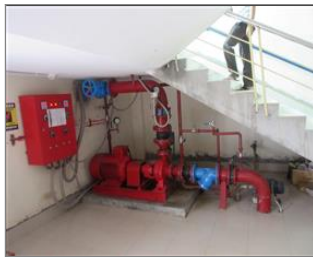
Photo of fire safety equipment Fire pump.JPG
