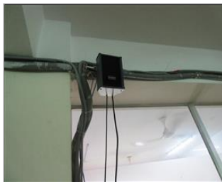
Photo of fire safety equipment PA System.JPG
