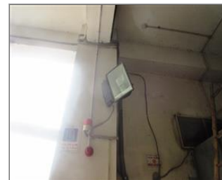
Photo of fire safety equipment Fire alarm.JPG
