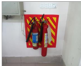
Photo of fire safety equipment Fire Extinguisher.JPG
