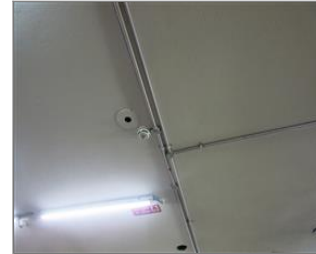
Photo of fire safety equipment Smoke Detector.JPG
