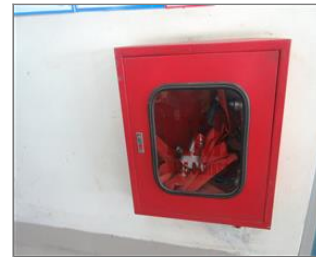
Photo of fire safety equipment Water hose pipe.JPG
